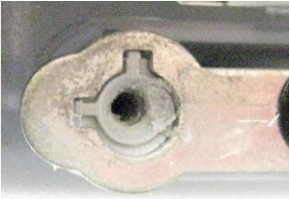
Fig. 3 Damaged screw hole.
